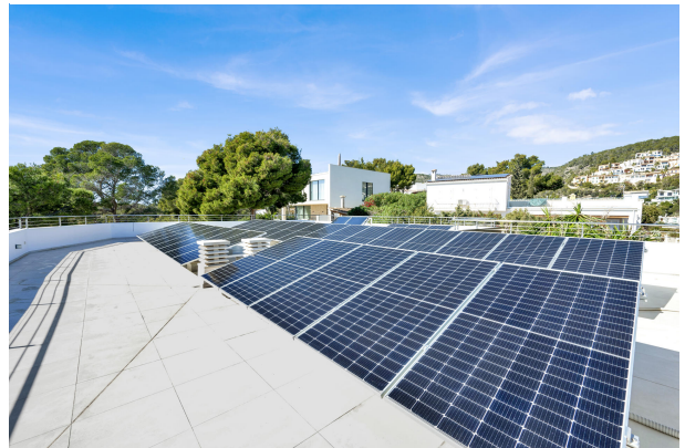
Solar panels on the roof terrace
