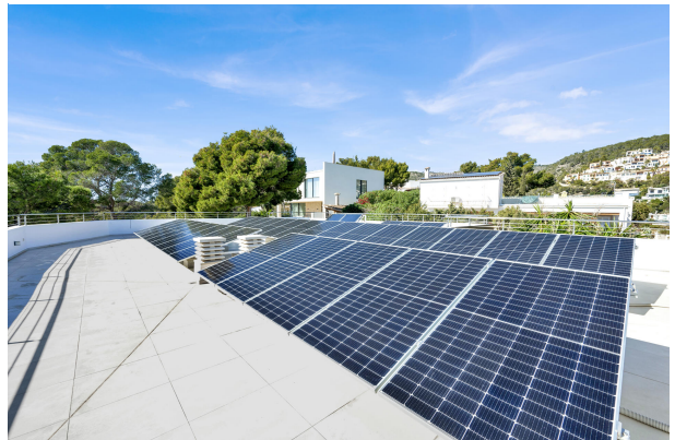
Solar panels on the roof terrace
